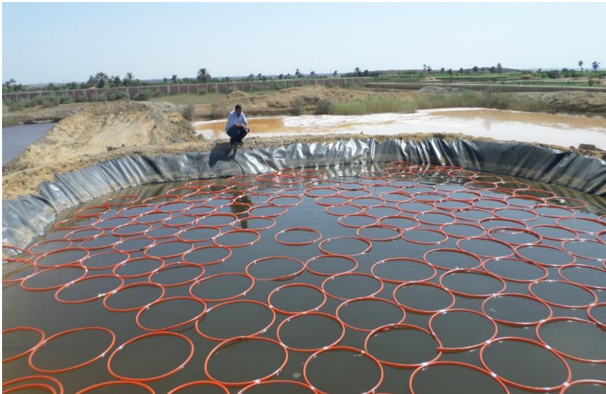
Figure 5: Implemented solar pond in Fayoum governate
